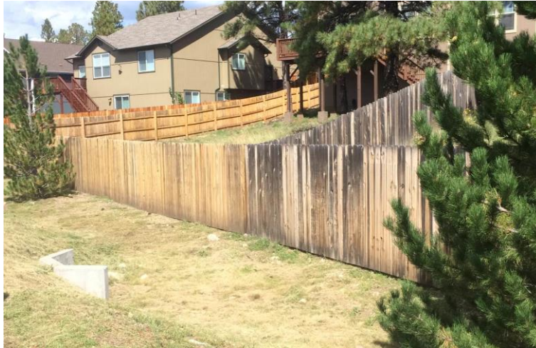
Figure 3.2.2: Fence slipping into the channel
